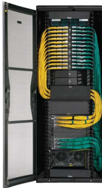
(Catalyst 6509 "Heavy Copper" Pre-Configured Physical Infrastructure shown)
